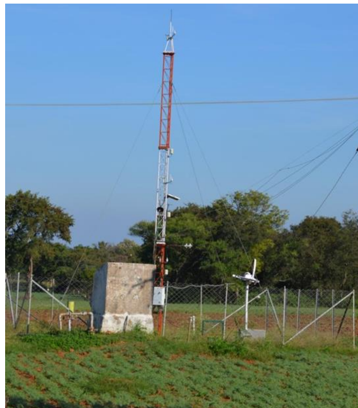
Figure 2-15: A typical AMS Tower Installed in the Field
