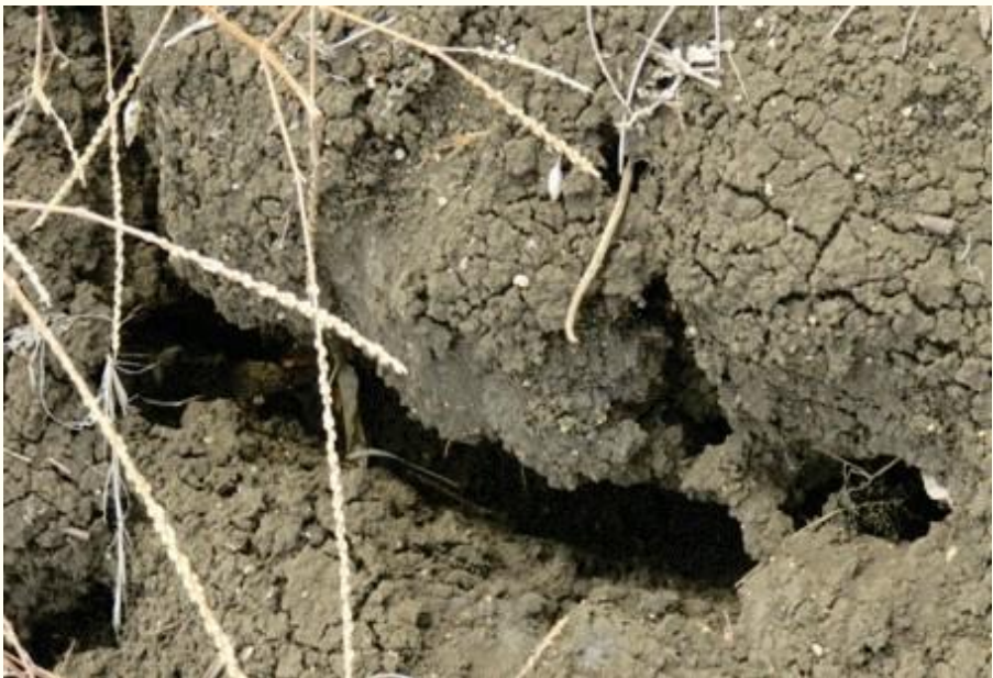
Fig 6.16 Deep and wide cracks on very gently sloping (1-2 % slope) uplands in S. No 52, Ladha 2 MWS, Kaudgaon village, Aurad Taluk, Bidar District
