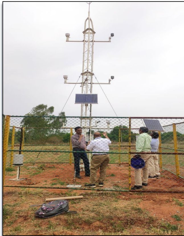
A typical AMS Tower Installed in the Field
